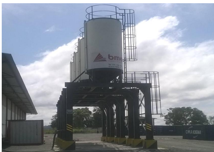
Figure 2.3-7: BME Storage Tanks (Silos)
